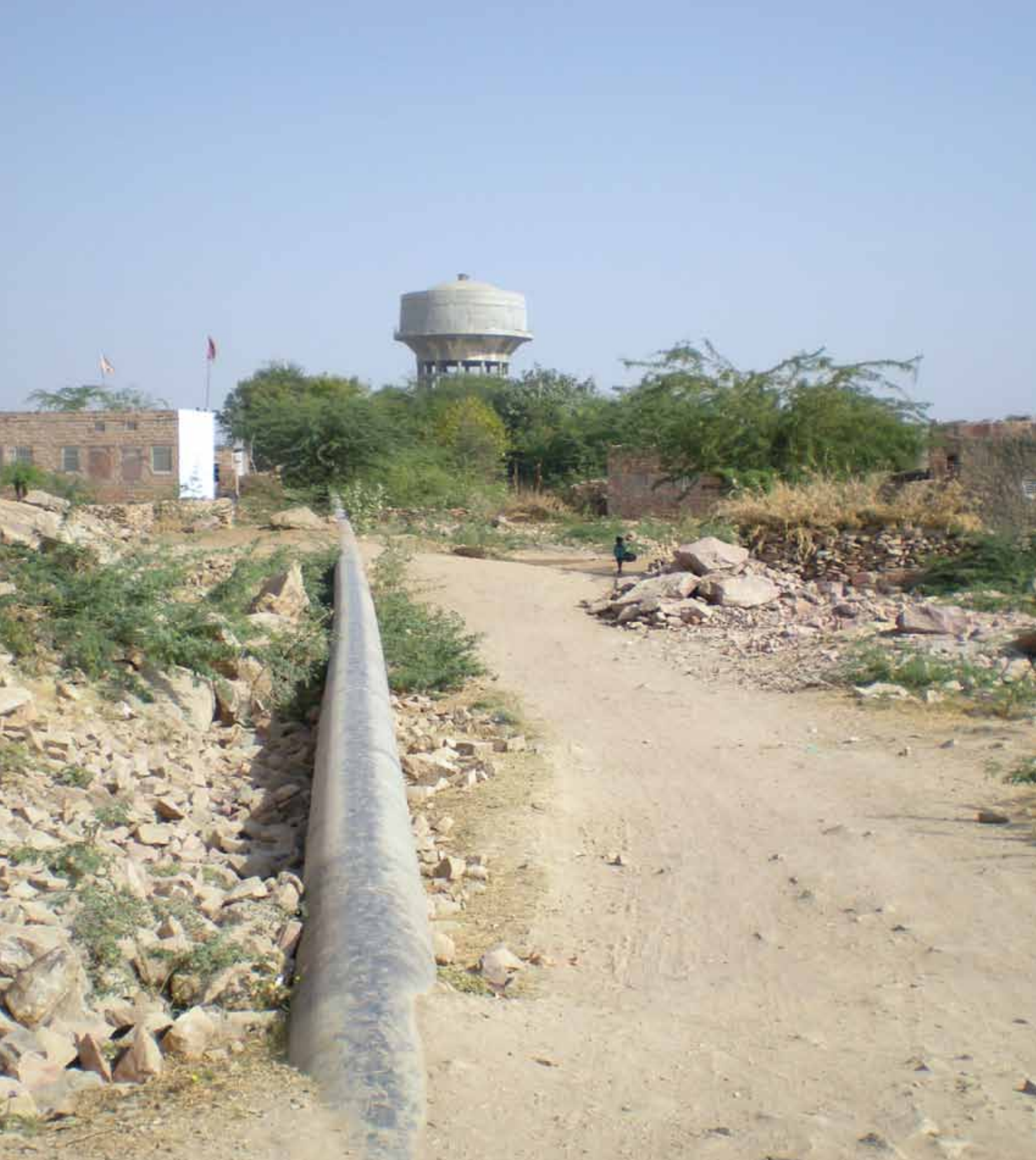
Jodhpur city water tank and pipeline running through the Kali Beri settlement
